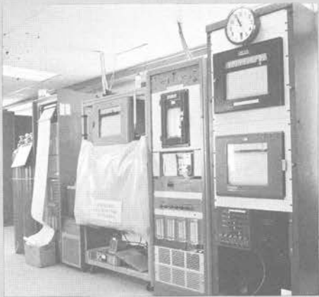
CO 2 instruments (left) in the new observatory building 1978, with meteorological and solar radiation strip charts (right).
