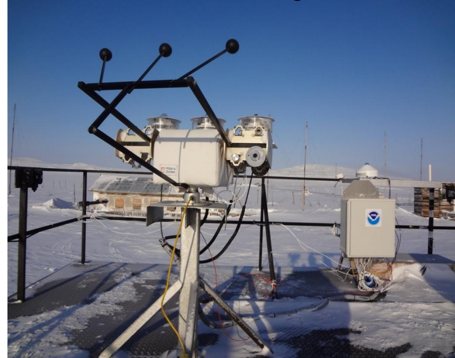
Sensors BSRN on the roof of HMO Main building
